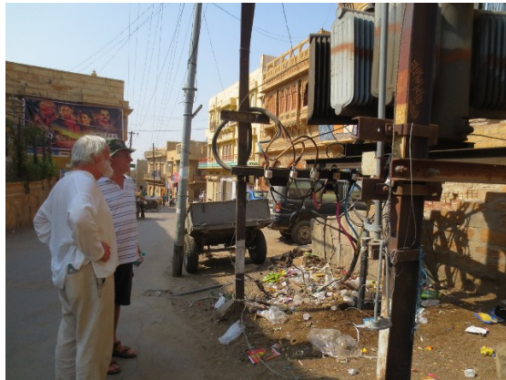
Rick and Peter checking out the dangerous wiring
