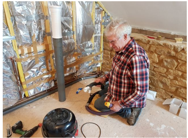
Rick dropped a piece of kitchen towel down waste pipe. He made a contraption that sucked it up from the garage 2 floors below
