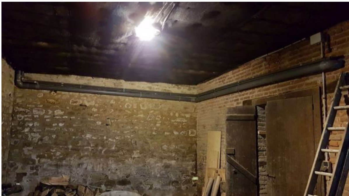
Plumbing and Electrics round the garage
