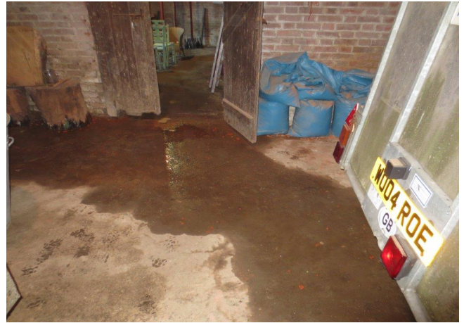
Water seeping through the garage floor
